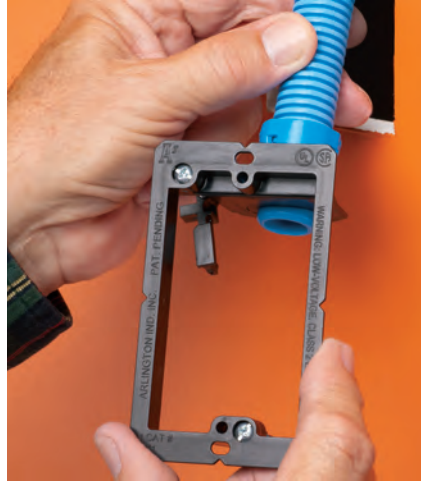
Insert tubing into the knockout.
